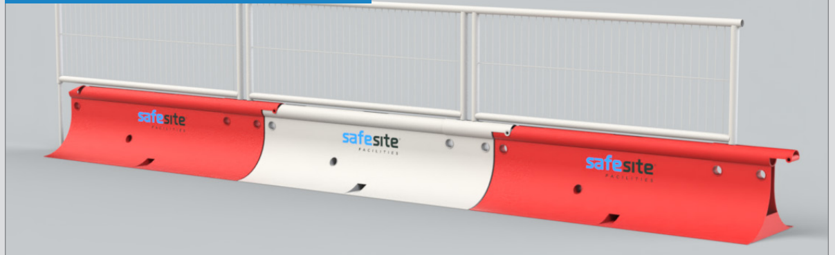
Row Of Bull Barriers With Pedestrian Fence
